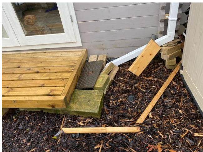
View of the drain within the rear garden of No.16 Conway Crescent (dated 25.08.20)
